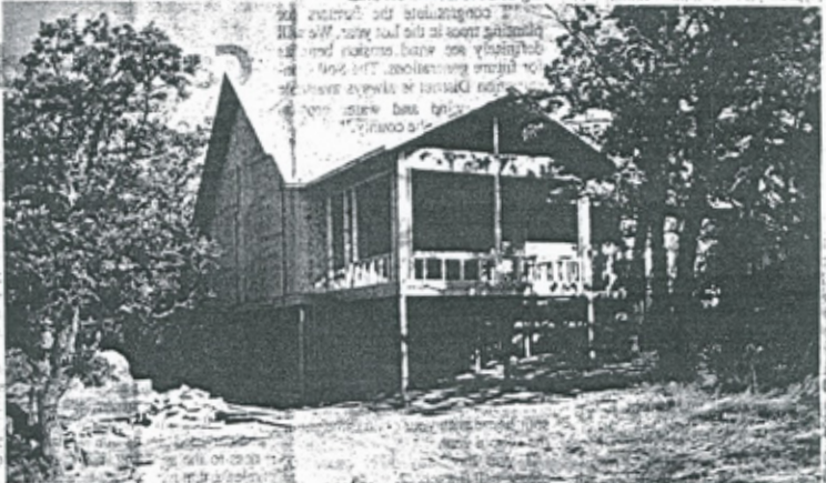
Under construction in Tiber Coulee is a cabin to be used for a Torgerson Family Retreat. It was Pete Torgerson's idea, but family and friends helped build it.
